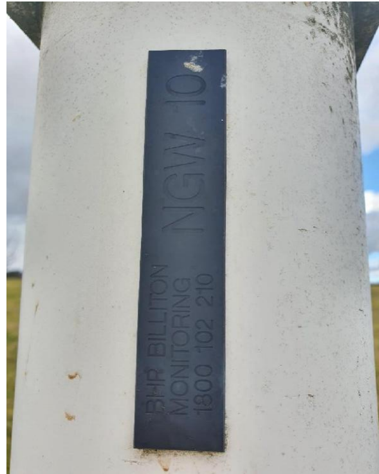
Photo 8 - BHP Monitoring Bore (MRP8)
