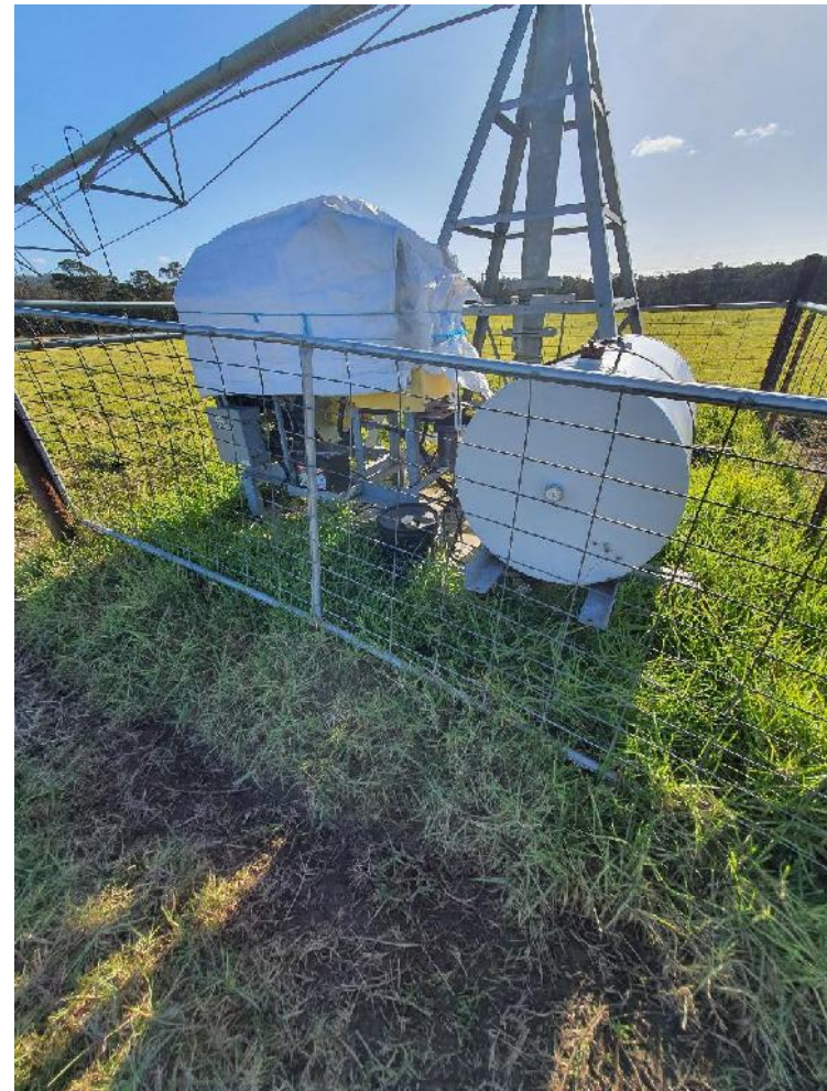
Photo 130 - Fuel Storage for Irrigation Pump (MRP114)
