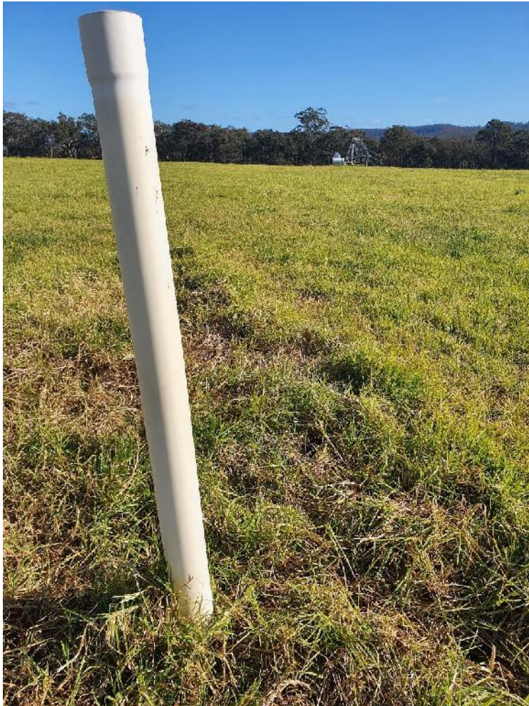
Photo 131 - Pipe Network for Irrigation (MRP115)
