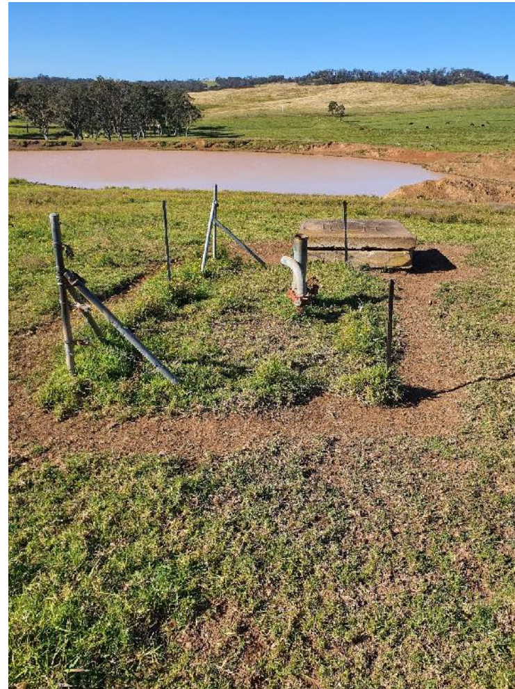
Photo 106 - Gas Well and Pipework (MRP94)
