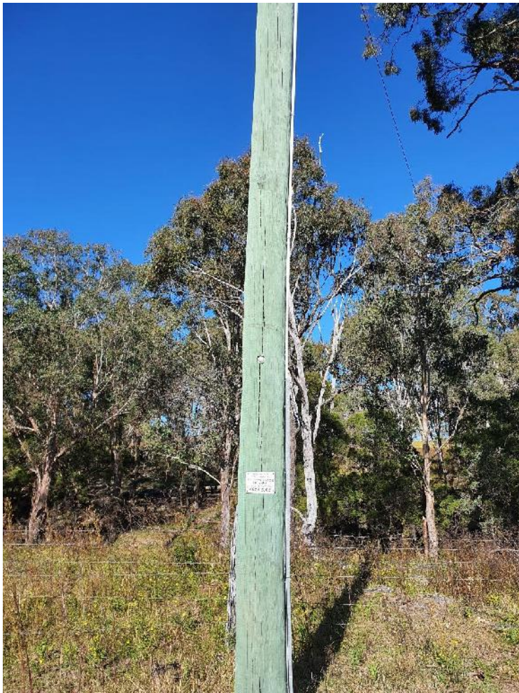
Photo 115 - Mine Communication Antenna (MRP100)
