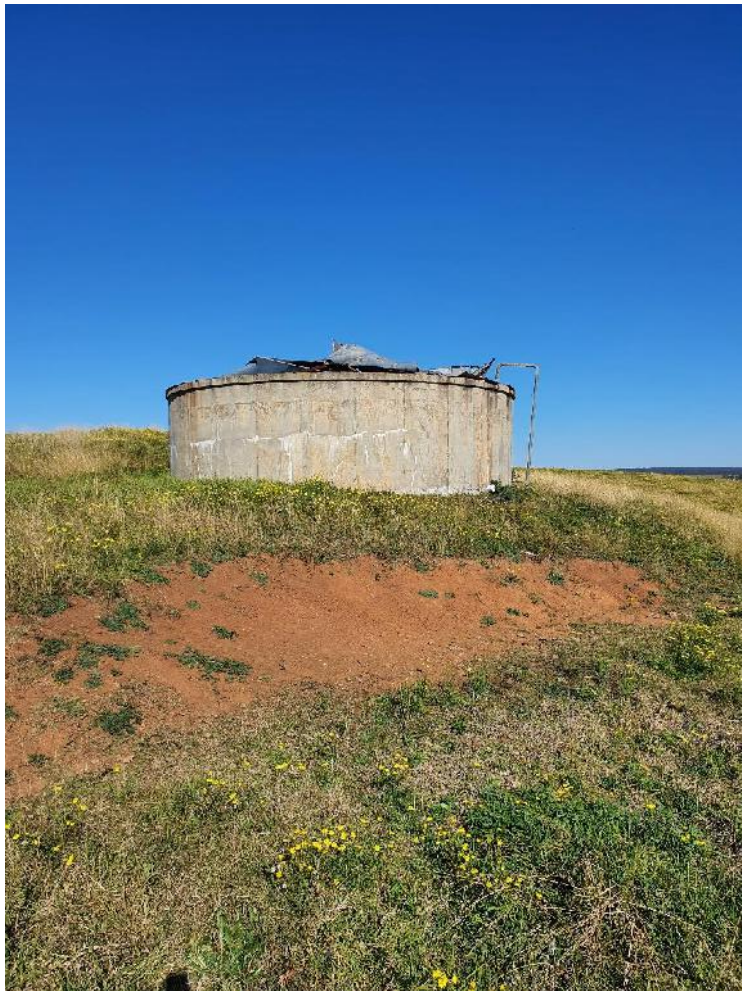
Photo 43 - Water Tank (MRP36)
