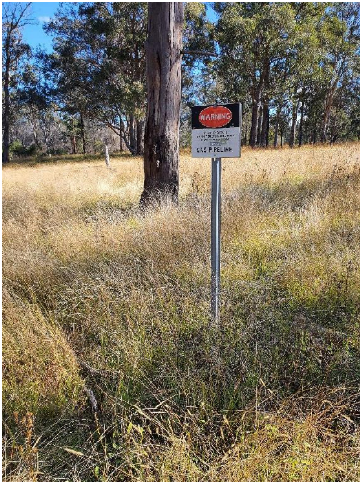
Photo 117 - Gas Pipeline (MRP102)
