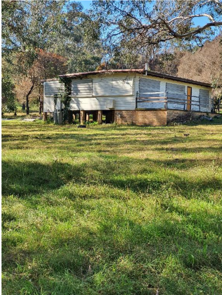
Photo 45 - Derelict House (MRP38)
