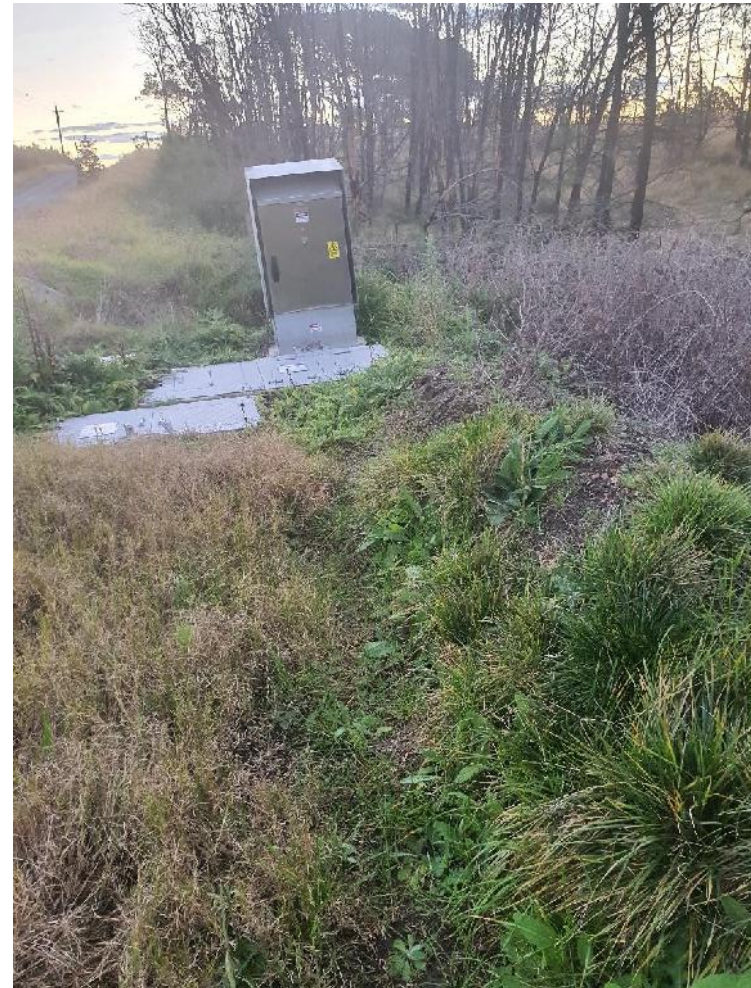
Photo 90 - Pump Station (MRP78)
