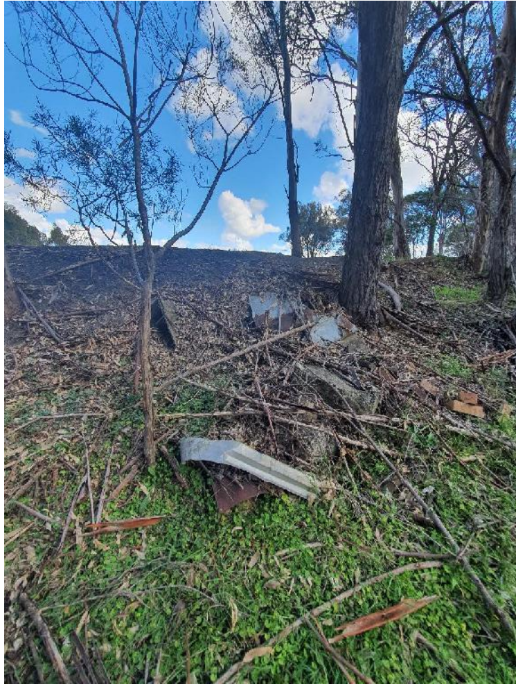
Photo 77 - Rubble in Dam Wall (MRP66)
